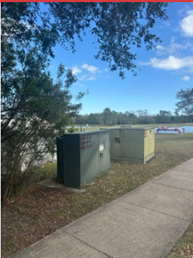
ELECTRICAL BOXES HAVE BEEN CLEARED OUT AT NO COST
