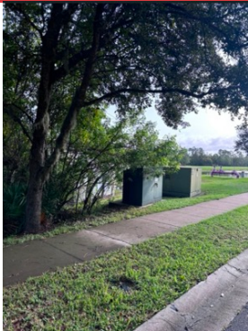
OVERGROWN WOOD-LINE ON ELECTRICAL BOXES
