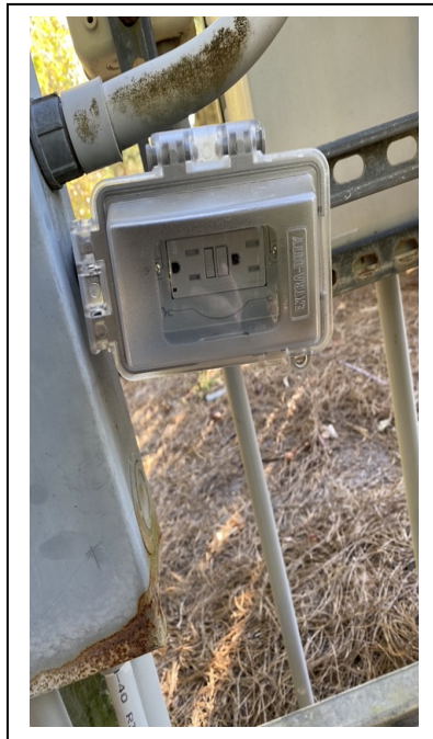
Future Horizons completed the Timer replacement to the fountain on US-1 and replaced the GFCI.
